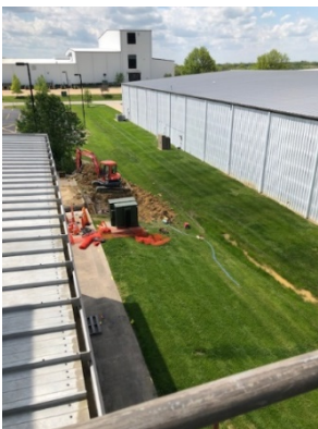
Installation of utility lines for the expansion of the University of Missouri Libraries Depository began in May. Photo by Kevin McFillen.
